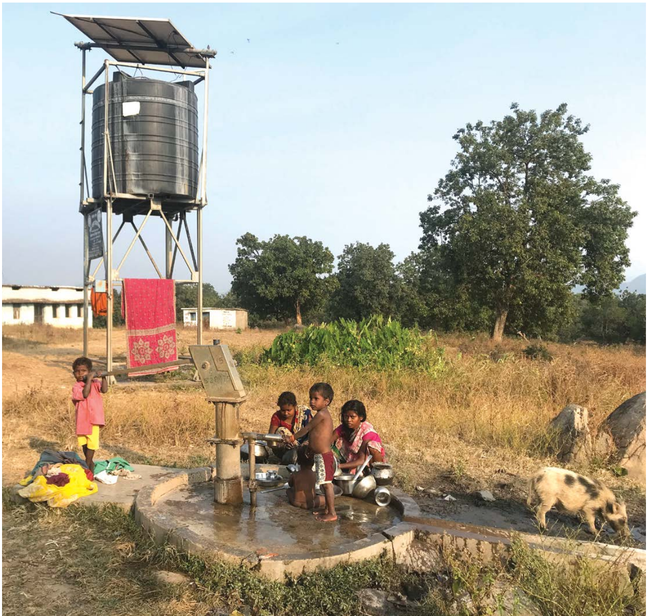
Solar handpump at a tribal village in Korba block/ Chinmayi Shalya, iFOREST
